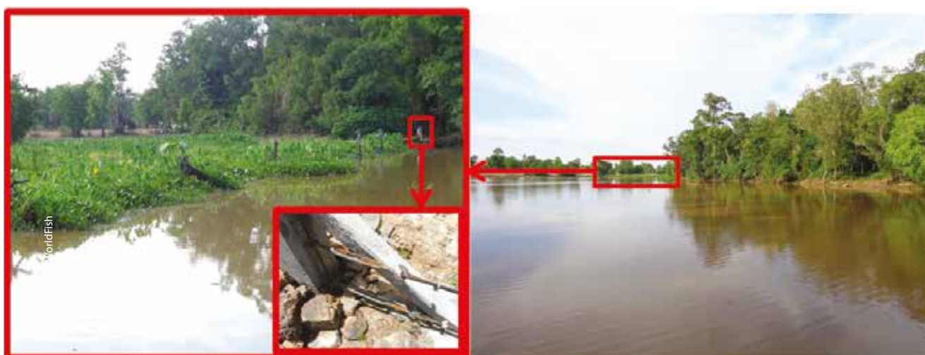
Installed cable to stop weeds from moving into CFR, Boeng Kampeng CFR, Pursat
