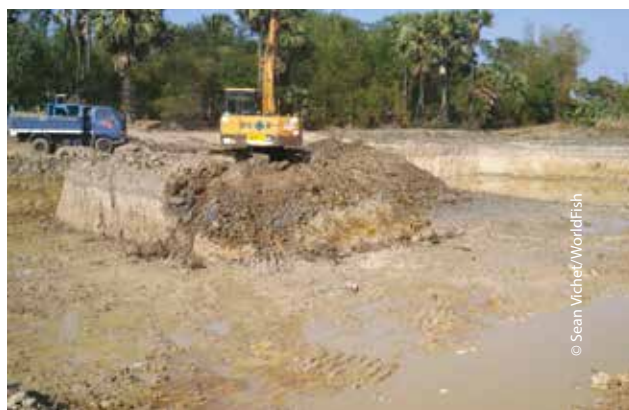
Deepening a part of a CFR to ensure it can retain water all year round, Boeng Tramses CFR, Pursat
